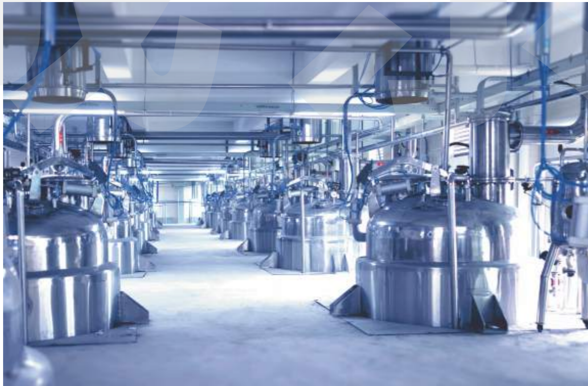
自动投料、加液系统 Auto Material Feeding, Auto Liquid Charging System
